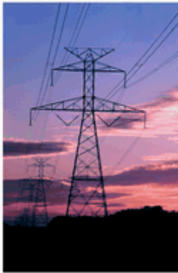
Oncor Electric Delivery
