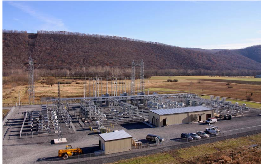
Example SVC Installation
