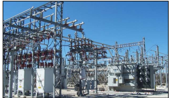
Pictured: Substation equipment
