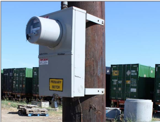
Pictured: Pole-mounted Meter
